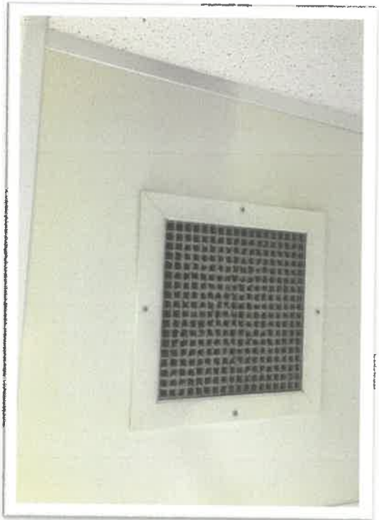
Photo O- Dirty Vent Common Area
