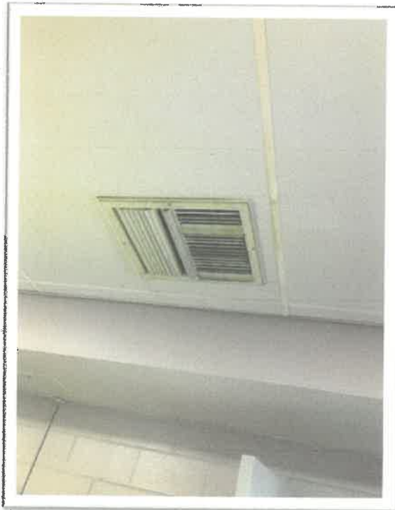
Photo H- Dirty Vent in Kitchen
