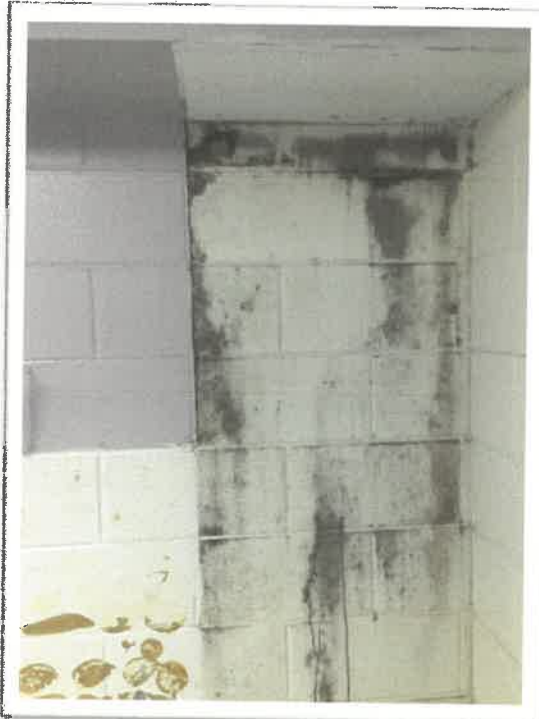
Photo A-Medical room-wall with mold
