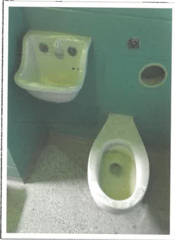
Photo E- Mod 1 Toilet Inoperable
