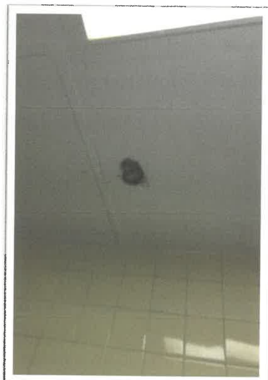
Photo L- Sprinkler Head Missing & gap
