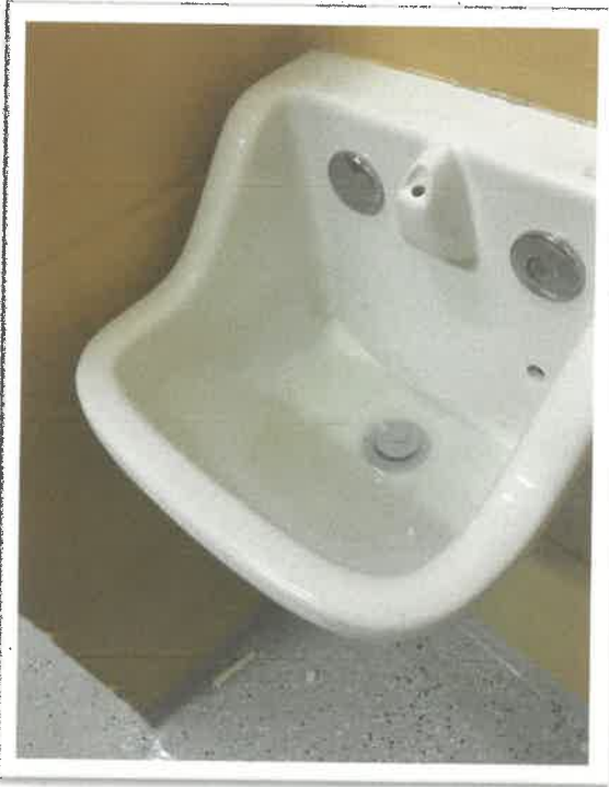
Photo B- Clogged sink room
