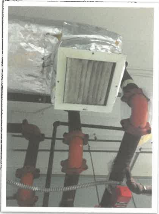
Photo N-Dirty Vent-Laundry Room
