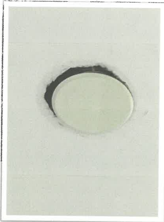
Photo M-Possible Missing Sprinkler
