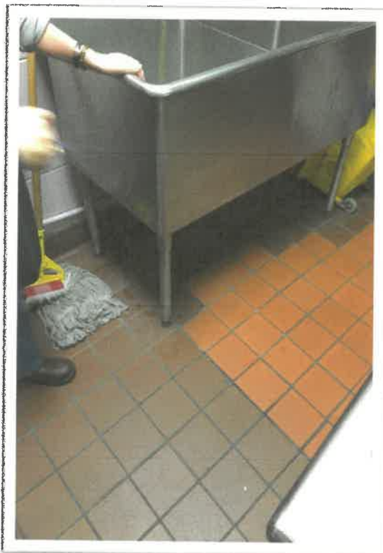
Photo K- Area where kitchen tiles lift
